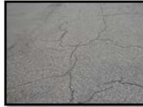
Transverse & Longitudinal Cracks
