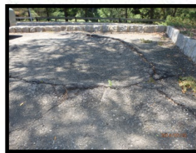
Upheaval of Pavement Surface
